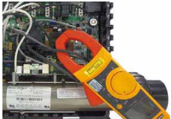
WHEN TESTING AMPERAGE
