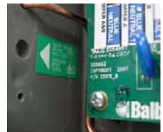
Ground in System Enclosure
